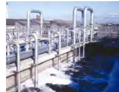
Wastewater treatment facilities
