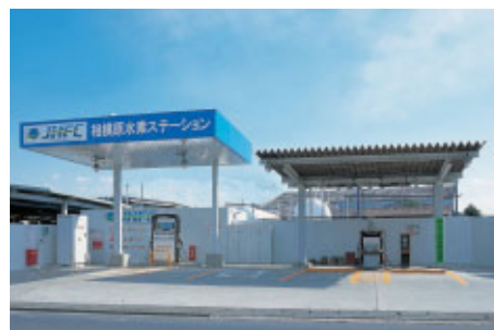
The JHFC station at Sagamihara, near Tokyo, is the world's first hydrogen fueling station utilizing mobile (truck-mounted) hydrogen production and compression facilities on the same site as an existing commercial LPG filling station.
