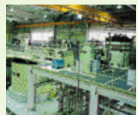
Wastewater Treatment Facility
