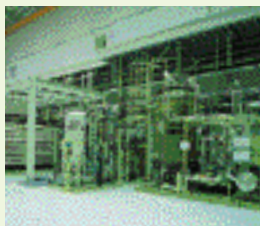
Ultrapure Water Production System
